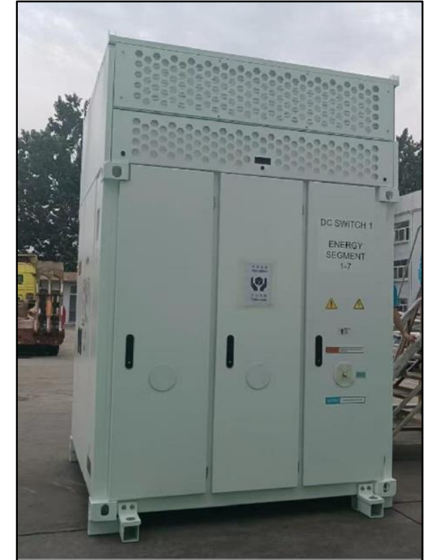
Lithium-ion battery unit example
