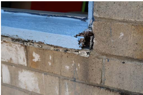
S35 – Rotting of the timber window frames of the storage building
