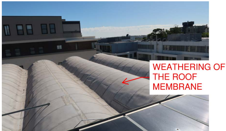
Figure 7 – Weathering of the Roof Membrane
