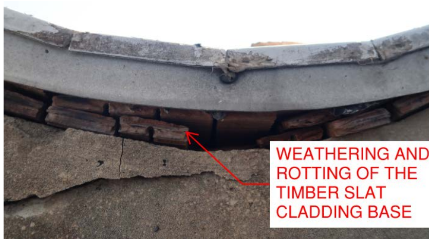
Figure 6 – Weathering of the Timber Slat Cladding Base
