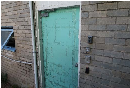
S31 – Damaged front entry door of the storage building
