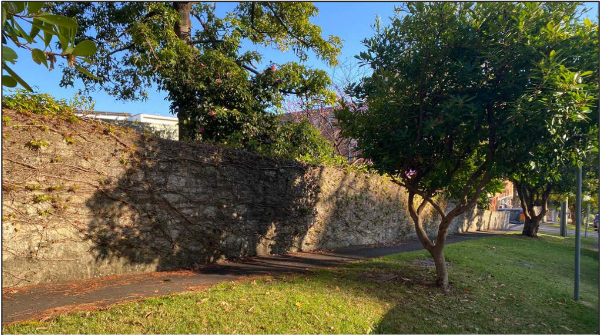
Figure 23 | Sandstone wall on Neringah Avenue South looking north-west from the south-east boundary of the site
