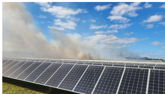
Grass fire burns under the solar panels
