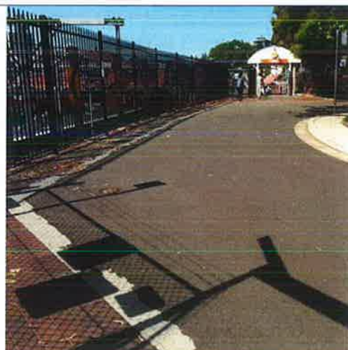
The brown brick is the narrow path on left leading short distance from ATP to Platform 10 entrance/exit. Grey area is Cornwallis St. The footpath is 0.73 metres wide.
